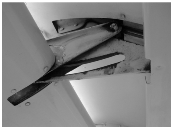
Check for damage to surfaces and flap tracks, freedom of operating linkage and security of all nuts and lock-wires.
