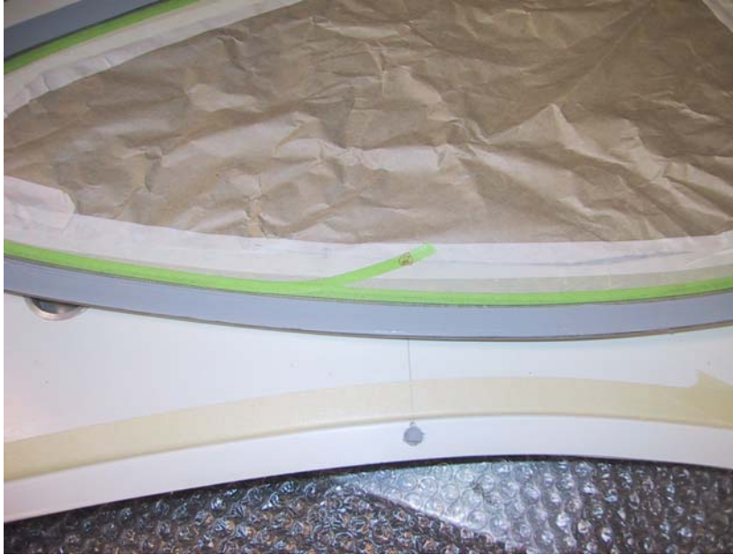
Figure A: Picture showing the taping details during the window installation process.
